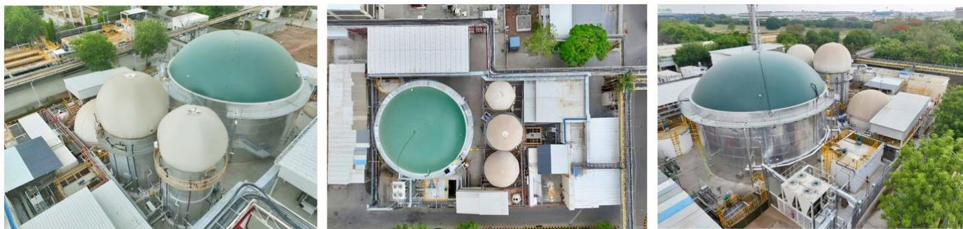
Aerial view of the biogas plant at Maruti Suzuki’s Manesar manufacturing facility
